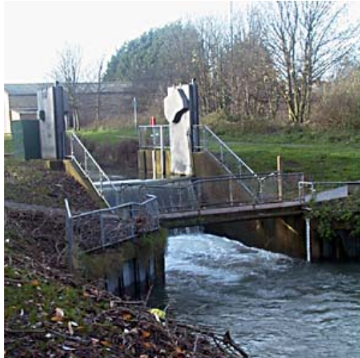
The Tilting Weir on the site of Town Lock - Louth
